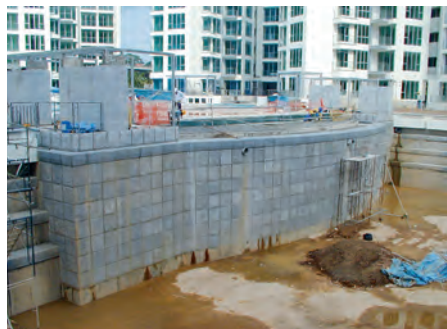
(From top) The waters beneath Corals at Keppel Bay (pictured) is an underwater sanctuary for King's Dock's thriving marine life. Precast granite slabs were installed onto the seawalls during the development of Keppel Bay to prevent erosion and seawater pollution.
